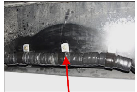
Ferrites installed on a cable harness
