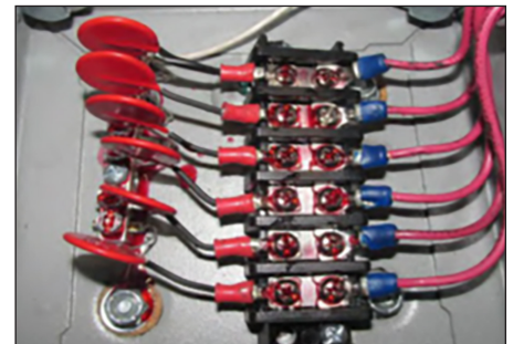
Tractor trailer terminal strip MOVs
